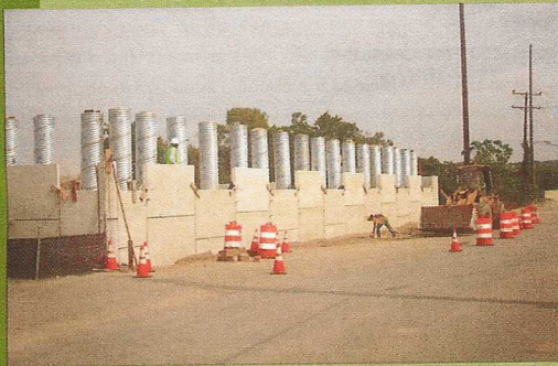
Northern wall under construction showing H piles inside the corrugated steel sleeves. Uses of sleeves gives the piles the necessary flexibility during expansion and contraction of the bridge without transferring those forces to the wall.
