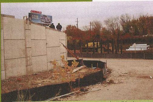
In the foreground is the completed North wall looking across Branchville Road at the piles that will support the bridge on the south side.
