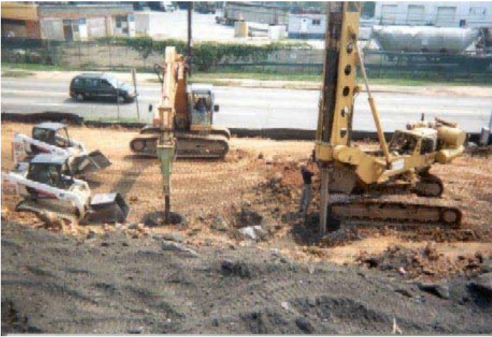
Geopier rammed aggregate piers were installed beneath spread footings in areas away from the Metro tunnel.
