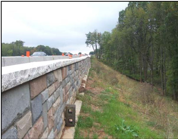
Undulating Wall & Slope failure
