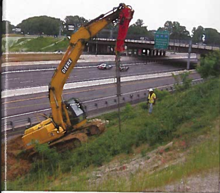
Small, mobile equipment allowed for work to be performed directly on the slope with no interruption of regular traffic patterns.
